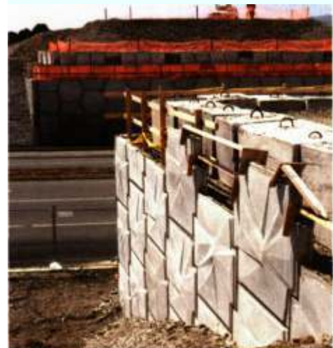
Mechanically Stabilised Earth (MSE) panelled walls located at Barrington Street form part of the Barrington Street Interchange. These panels are created to visually represent the incised and buckled forms of the Southern Alps.
