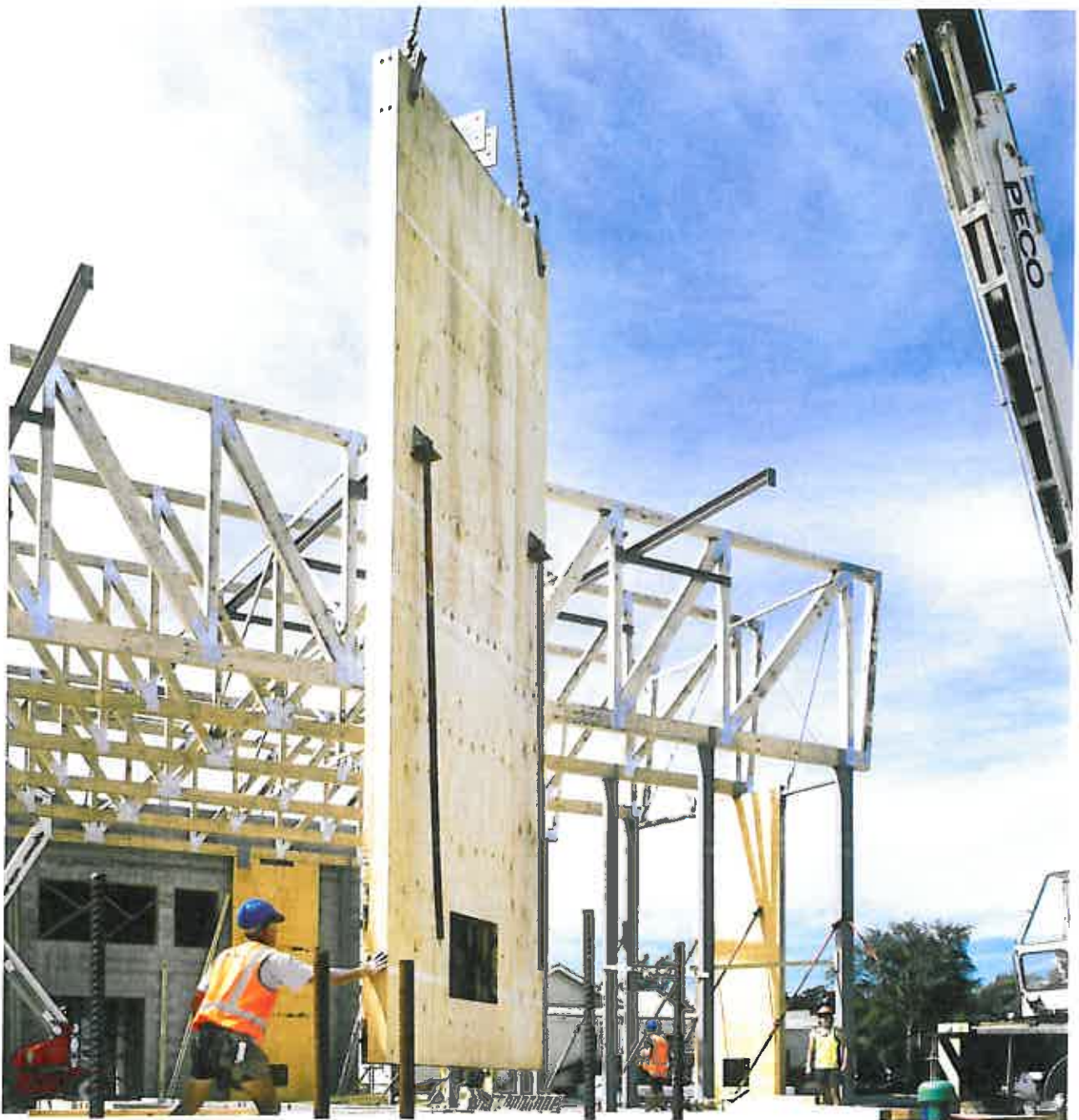
The steel ball of the crane is used to lift the timber panel into place. A team of workers are working together to push the panel into place.
