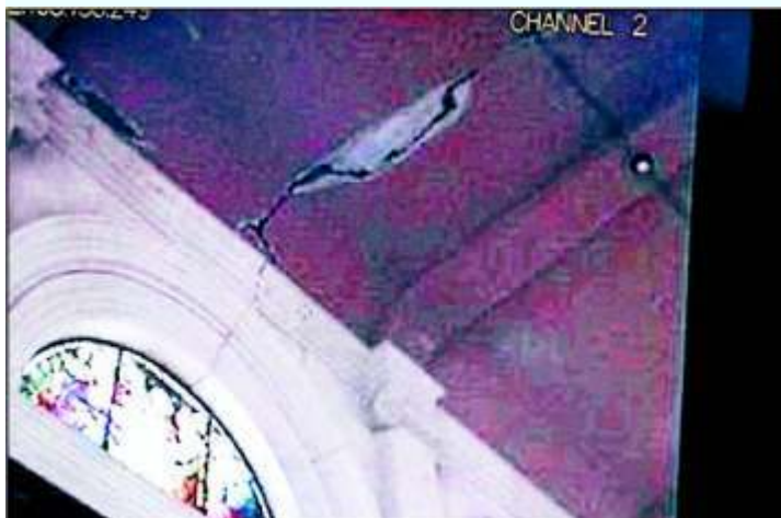
Filming the devastation: The robot supplied the first clear pictures of the inside of the cathedral since the February 22 quake.
